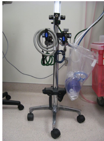
Image 2: Mobile gas delivery system in dental office/clinic
