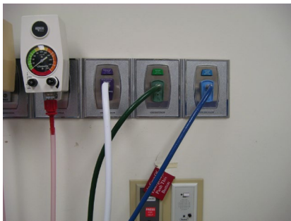
Image 1: Gas lines from wall in dental office/clinic
