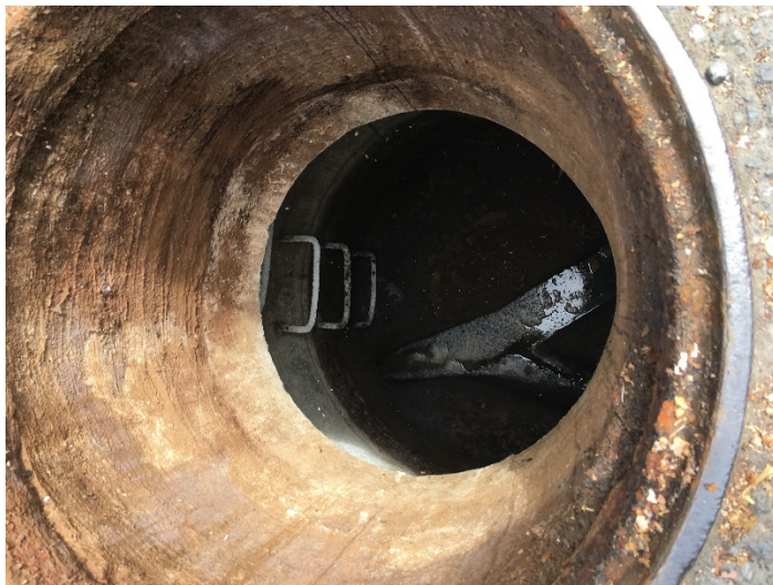
Figure 27: Entry to manhole. Note manhole steps start some distance from opening. Fall protection is critical upon entry.
