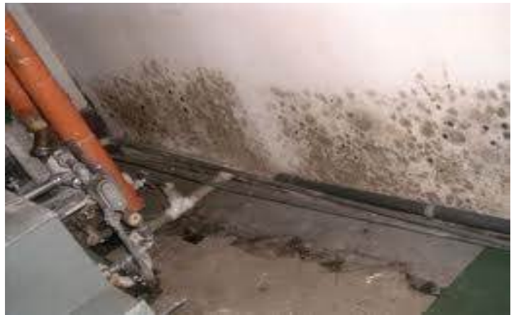
Major mold growth in cold room mitigated by UW Facilities' contractors
