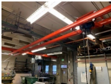
Figure 1: Double girder bridge crane with trolley mounted underneath
