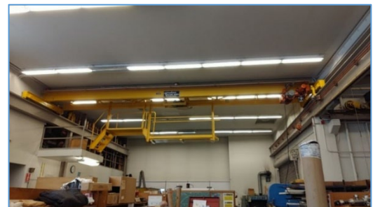
Figure 2: Double girder bridge crane with trolley mounted on top of girders
