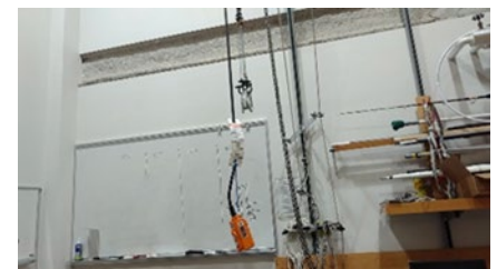
Figure 13: Pendant Controls (UW installation)
