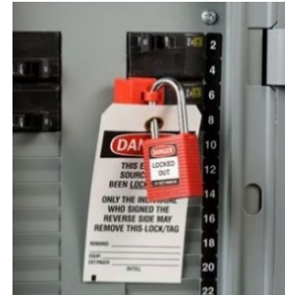
Circuit breaker lockout device locked and tagged out Brady.com
