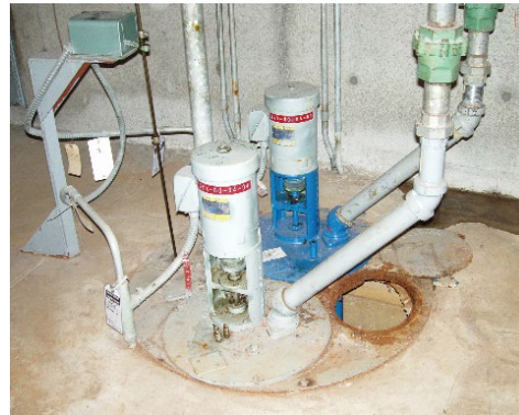
Sump pumps (electrical and hydraulic)
