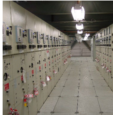
Electrical switch gear room
