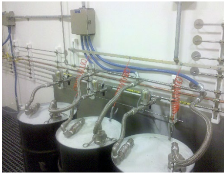
Chemical – flammable solvent dispensing system
