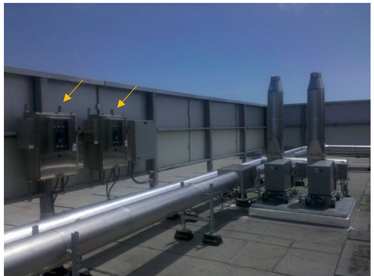
Exhaust fans and motors with accessible local disconnects
