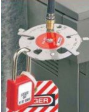
Locked compressed air line
